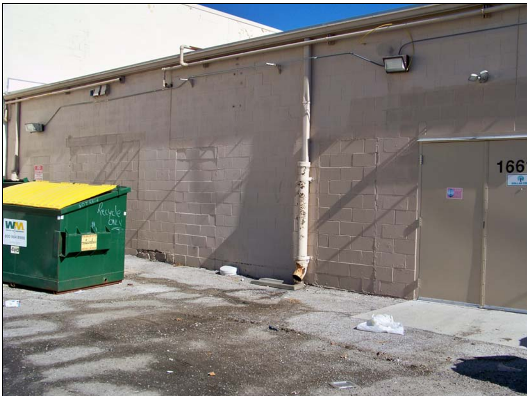
Building 1 – looking east – deterioration of wall, gas line, downspout, pavement
