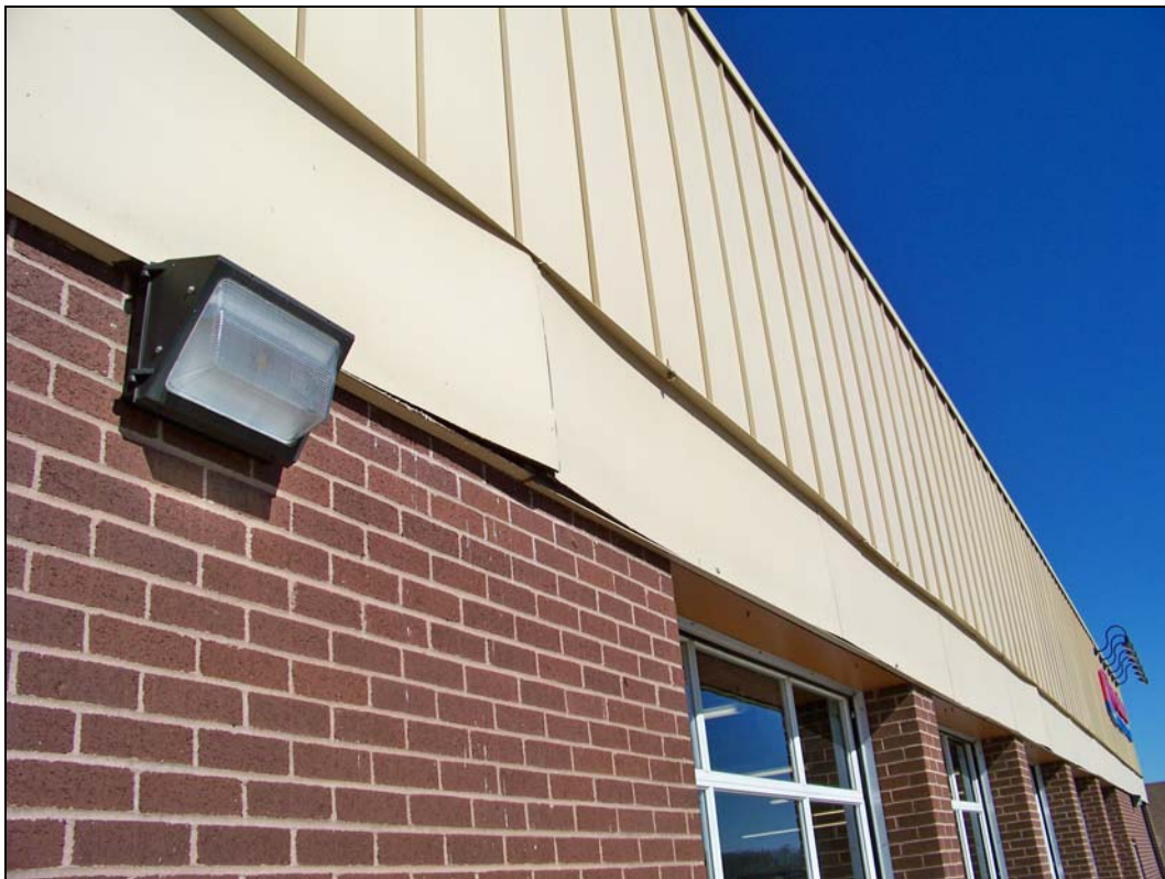
Building 3 – looking northeast – deterioration of fascia, siding
