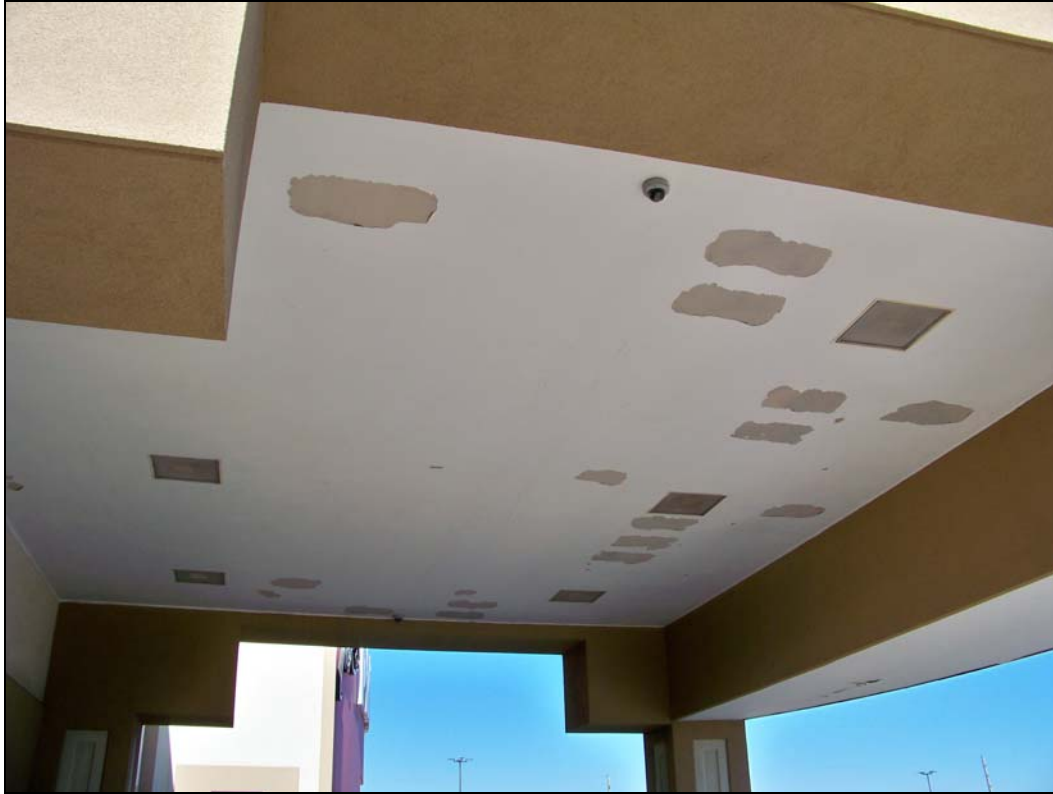
Building 1 – looking north – deterioration of soffit; failure of finishes
