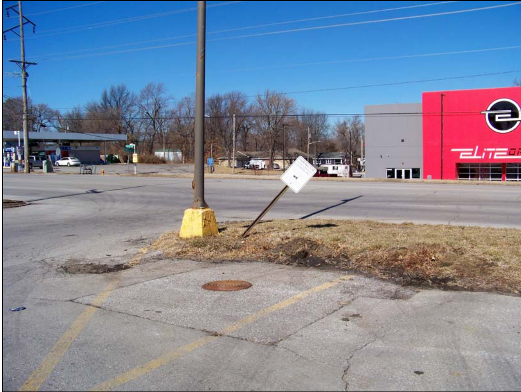
Near Building 1 – looking northwest – deterioration of pavement, curb, signage; damaged landscaping
