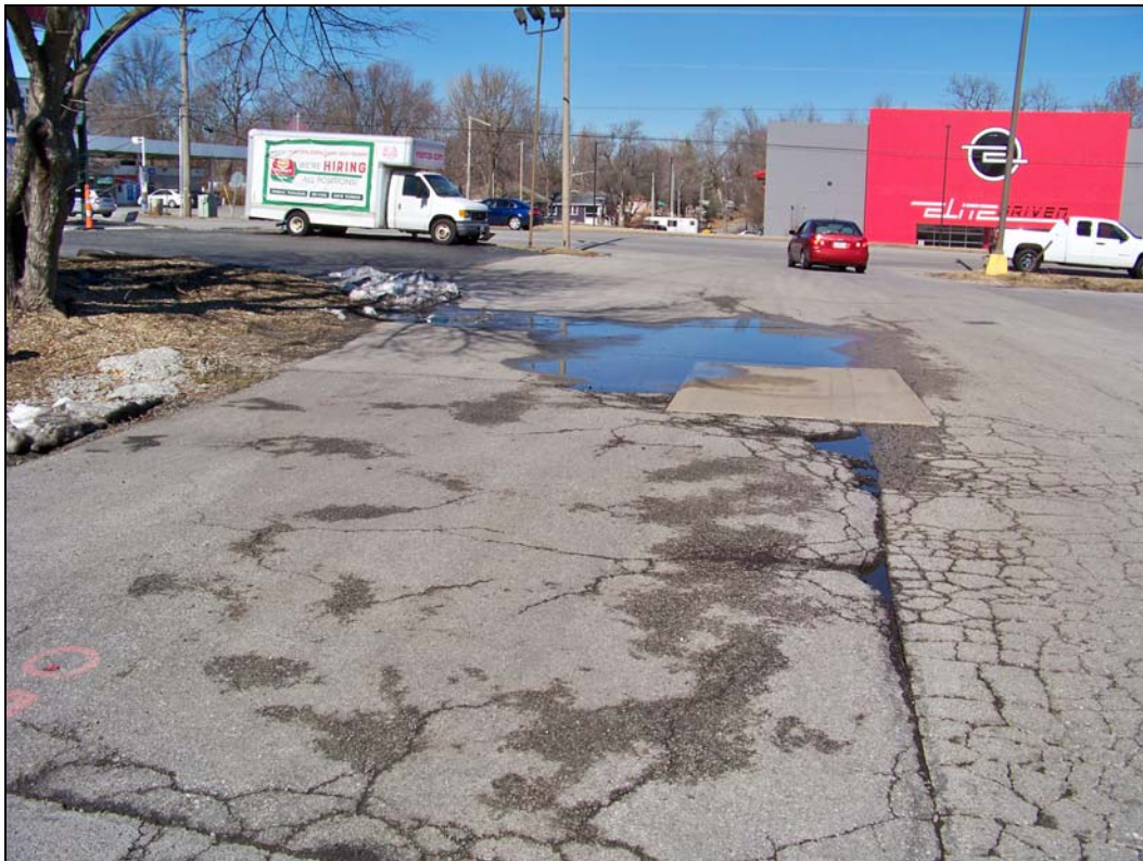
Near Building 1 – looking north – deterioration of drive aisle; poor drainage
