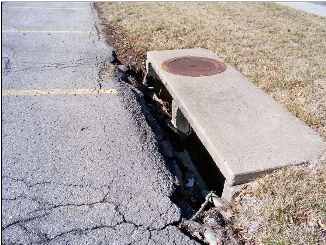
Near Building 1 – deterioration of stormwater basin
