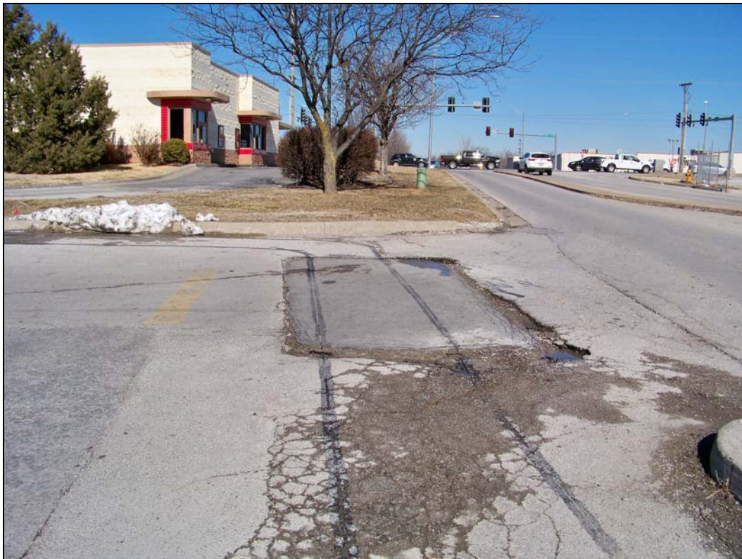
South of Building 2 – looking north – deterioration of pavement
