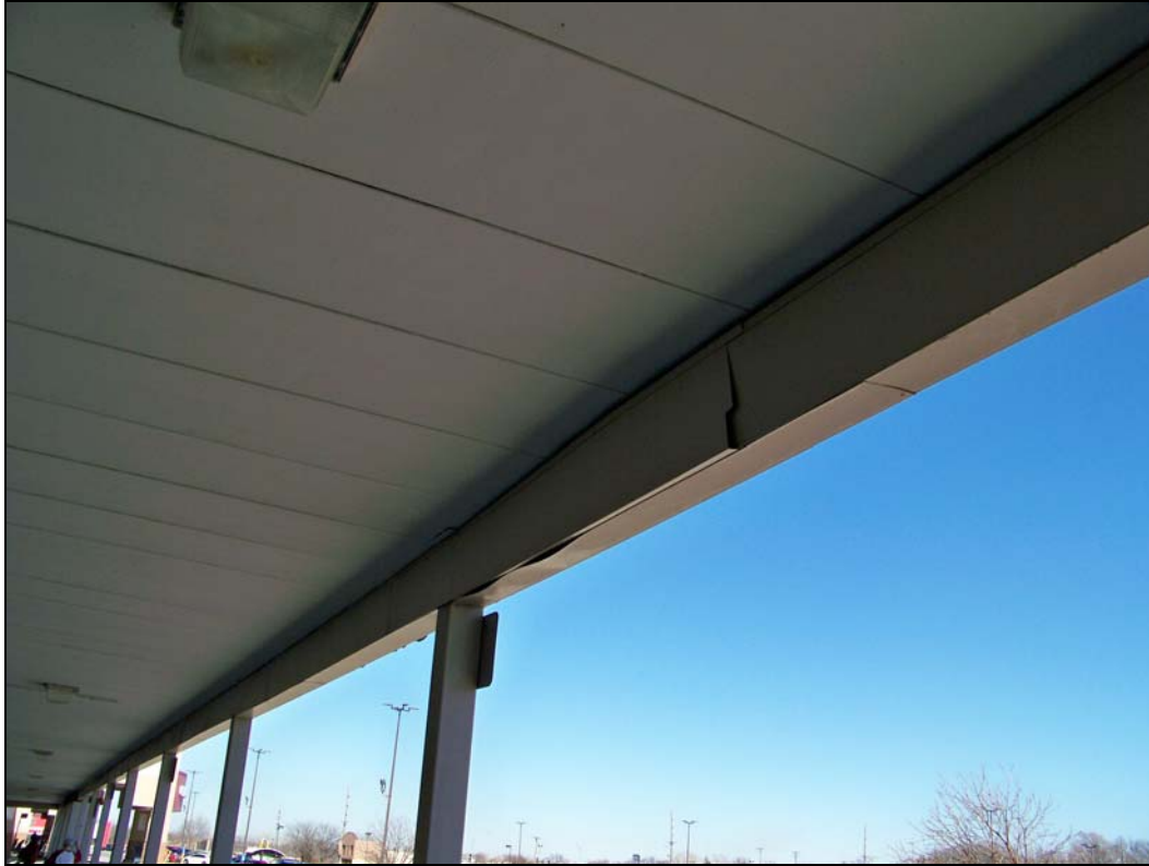
Building 1 – looking north – deterioration of canopy beam and fascia
