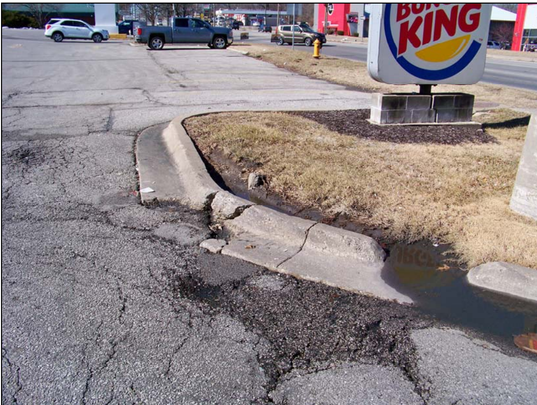
Building 3 – looking west – deterioration of sign, curb, drive aisle; damaged landscaping
