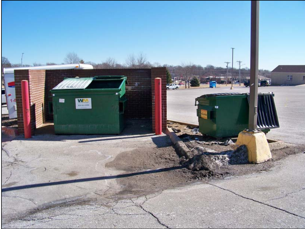
Near Building 3 – looking southeast – deterioration of trash enclosure, parking lot and island
