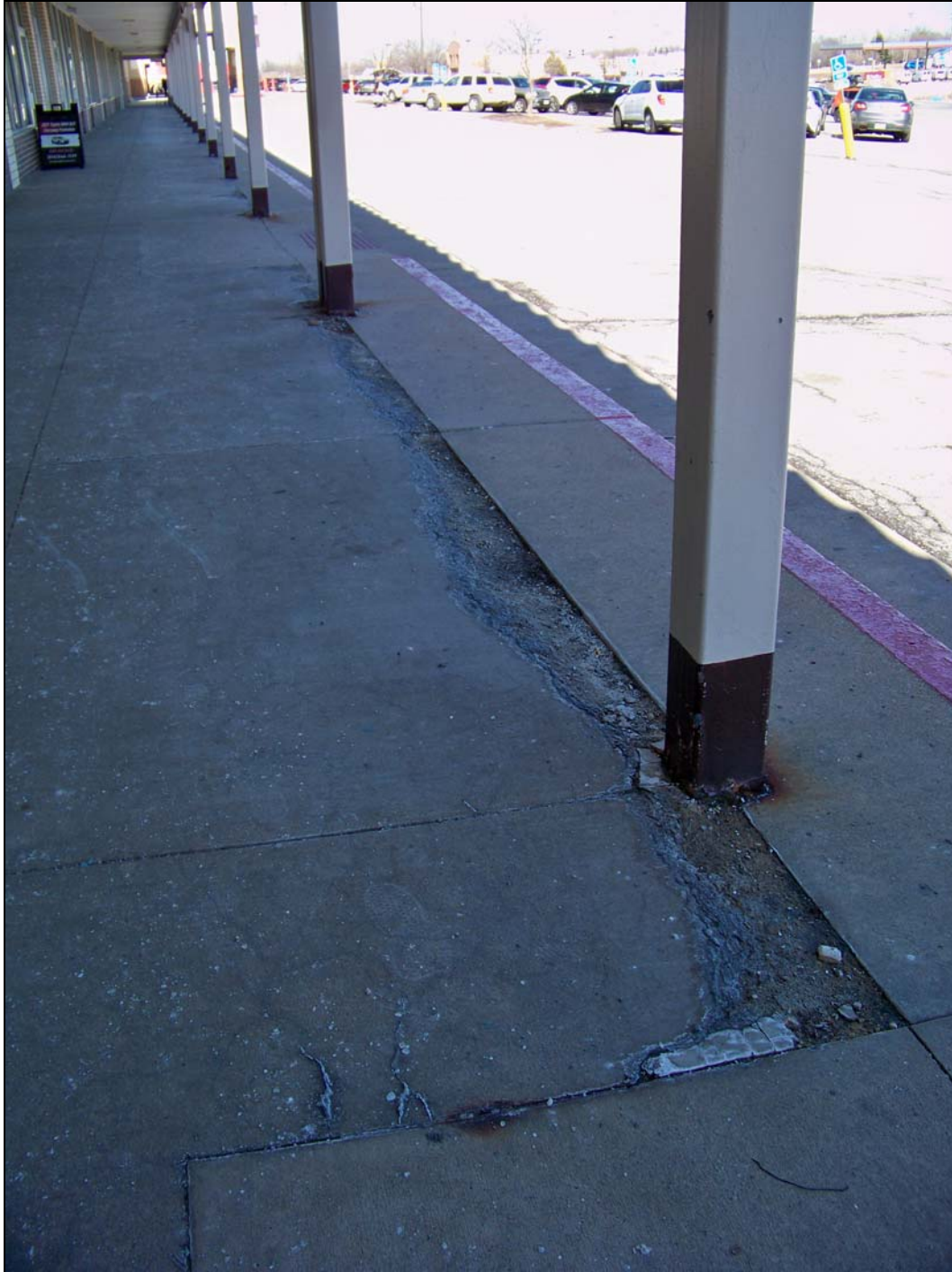
Building 1 – looking north – deterioration of canopy columns, sidewalk
