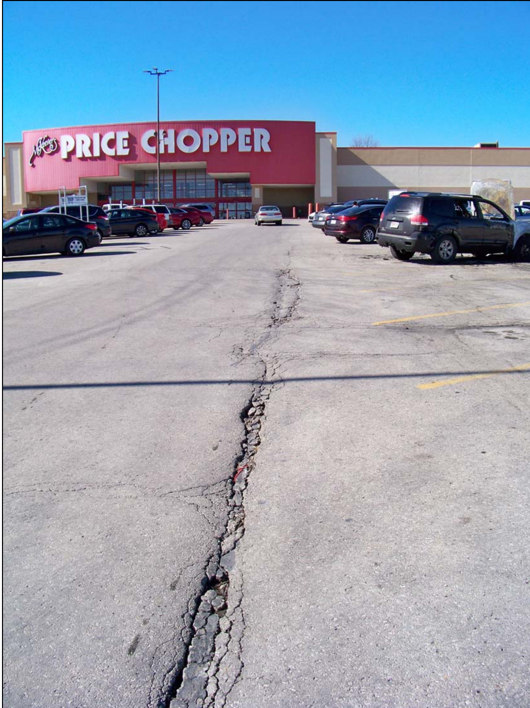
Building 1 – looking west – deterioration of pavement; burned-out vehicle
