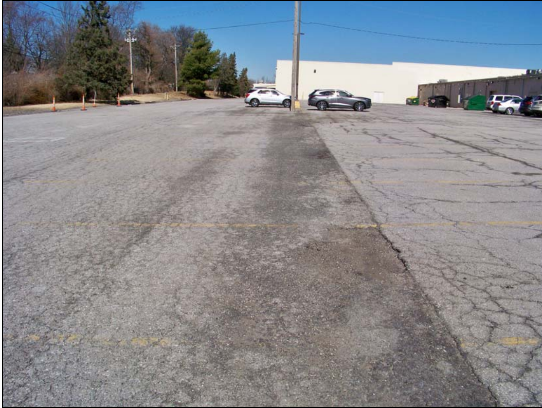
Near Building 1 – looking north – deterioration of pavement
