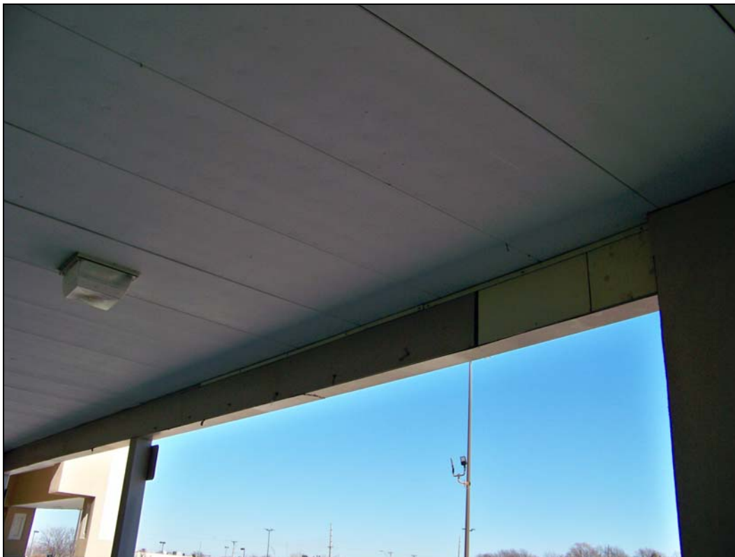
Building 1 – looking northeast – deterioration of canopy beam and fascia
