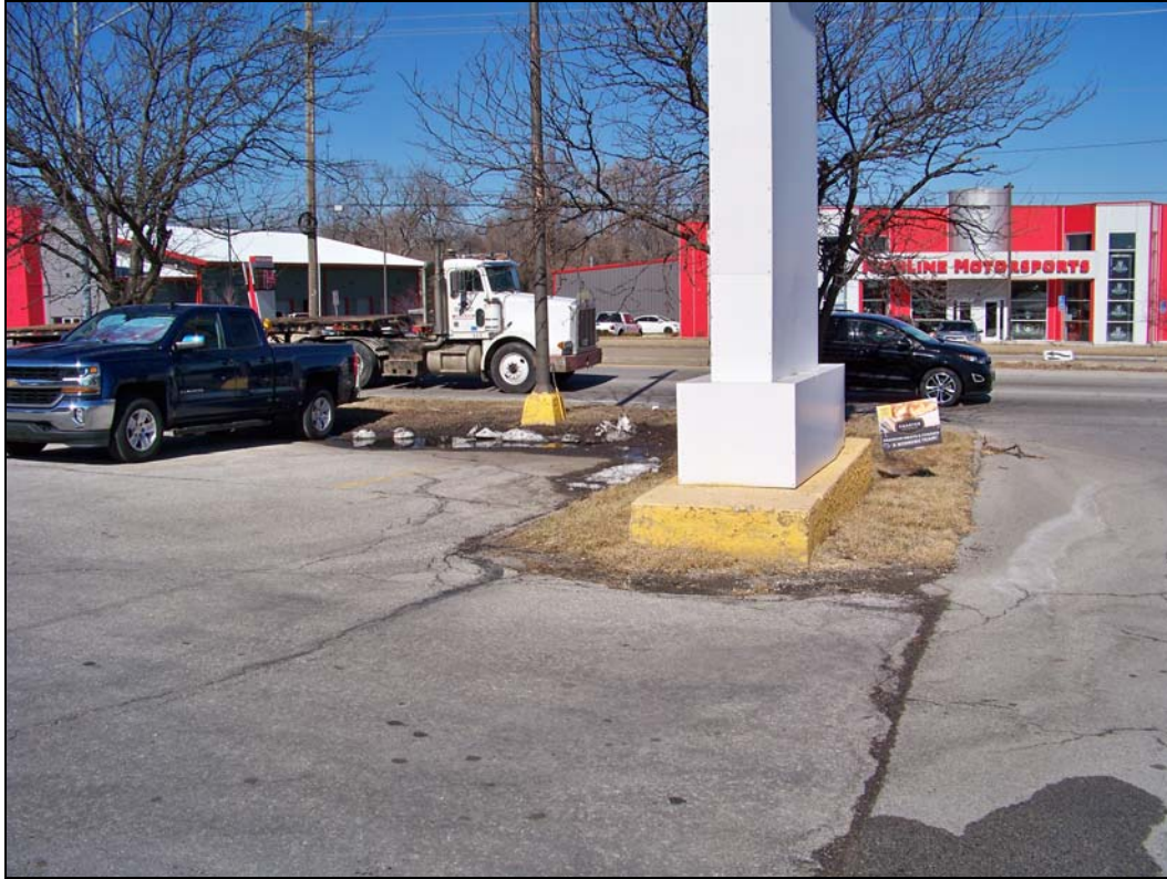
Near Building 1 – deterioration of curb, parking lot; poor drainage
