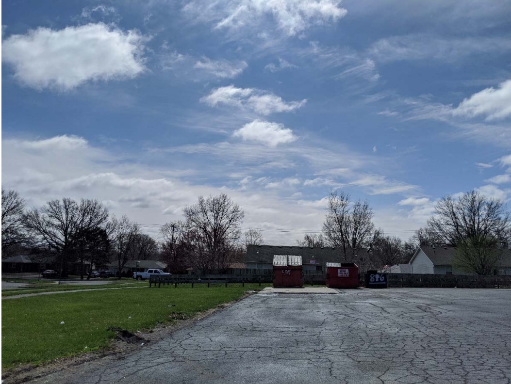
Deterioration of parking surfaces; Trash/debris
