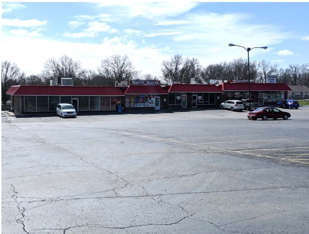
Deterioration of parking surface
