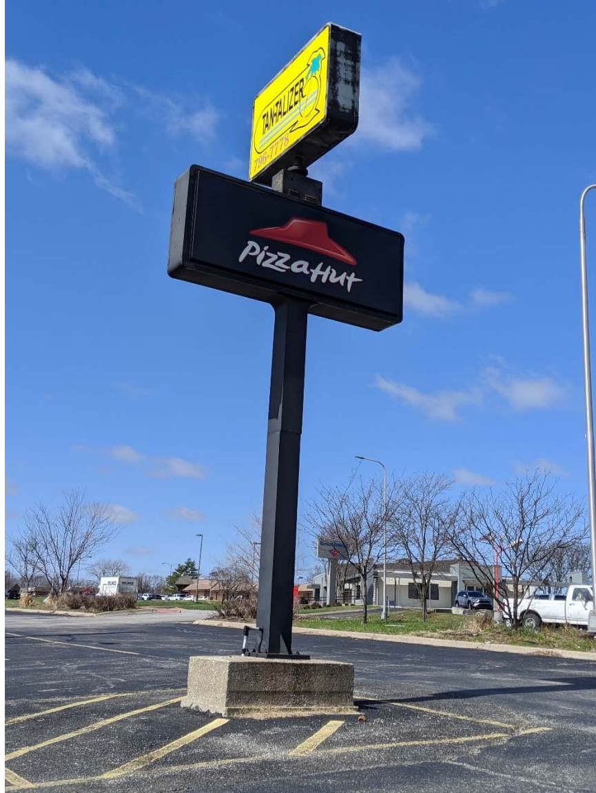
Deterioration of sign
