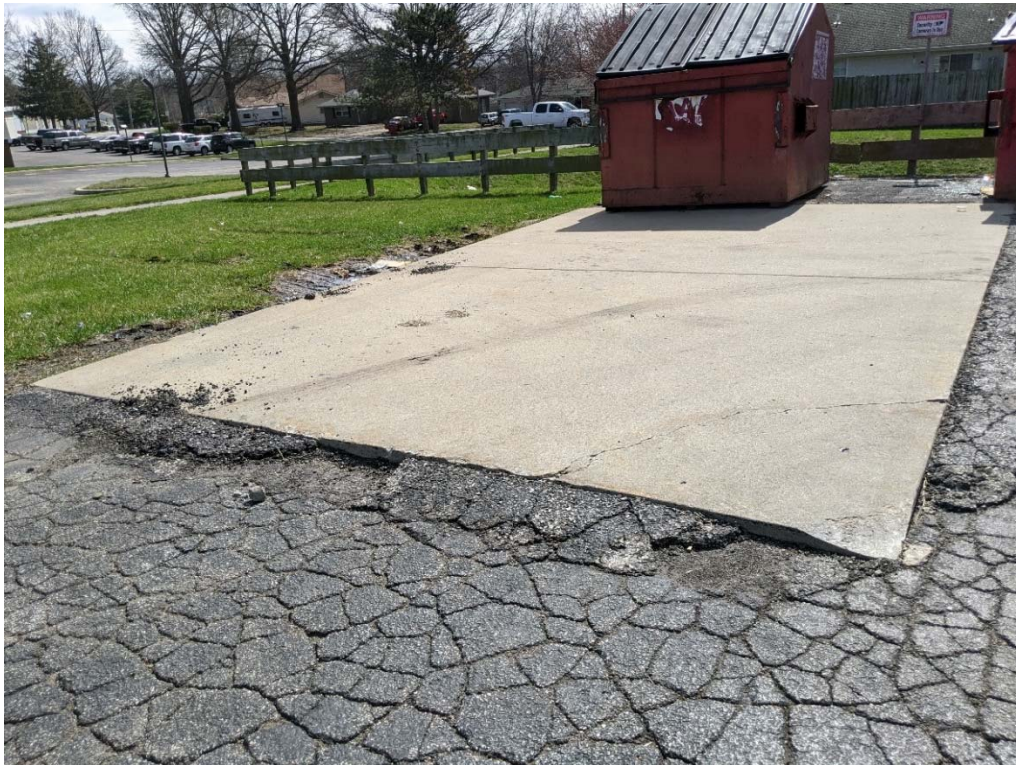
Deterioration of drive; unscreened trash areas
