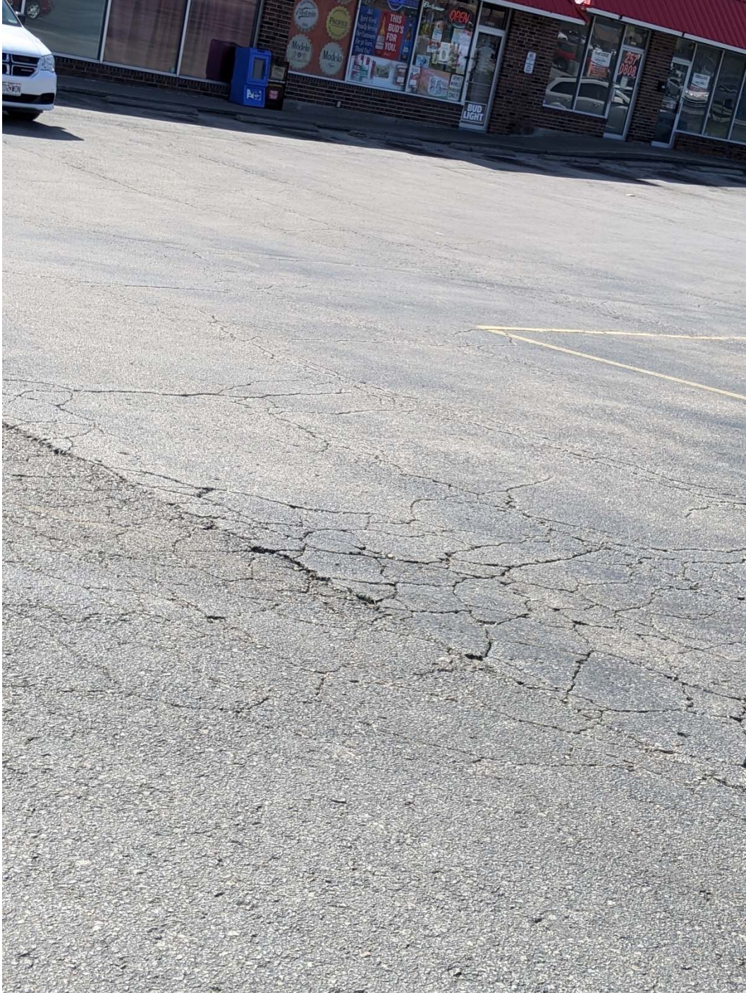
Deterioration of parking surfaces
