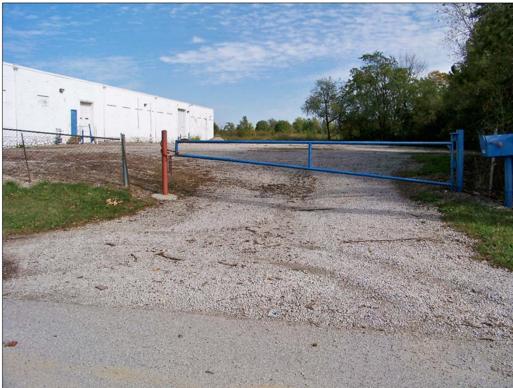
Deterioration of driveway at Weatherford Ave. building
