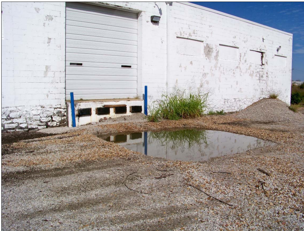
Failure of finishes, deterioration of windows, poor drainage, trash/debris at Weatherford Ave. building
