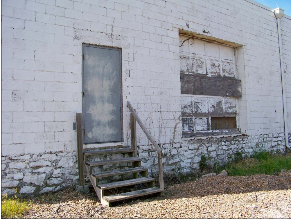
Failure of finishes, deterioration of doors and steps at Weatherford Ave. building
