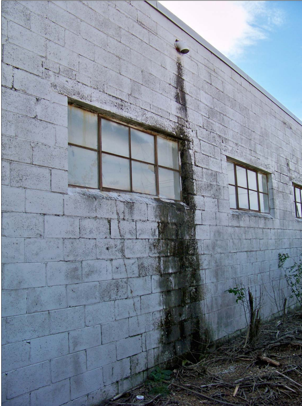
Failure of finishes, mold/fungi growth, deterioration of windows at Weatherford Ave. building
