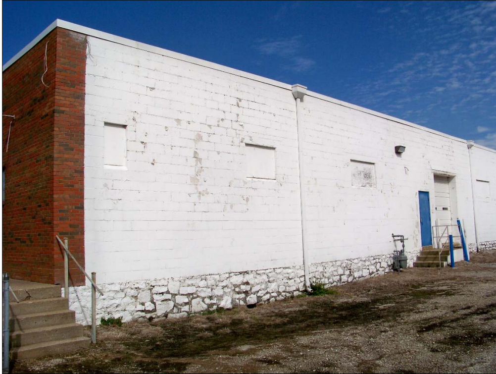
Failure of finishes, deterioration of windows at Weatherford Ave. building
