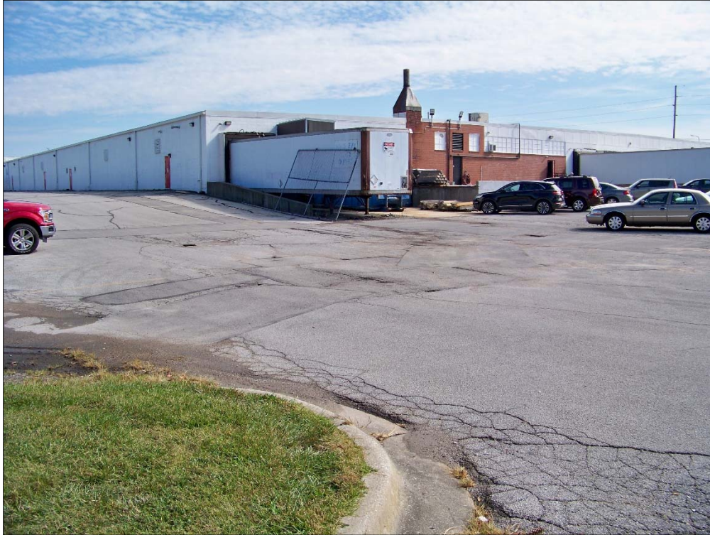
Deterioration of parking lot at Cargo Largo building
