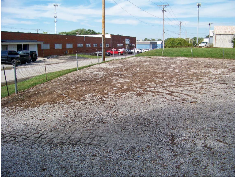
Deterioration of surface parking at Weatherford Ave. building
