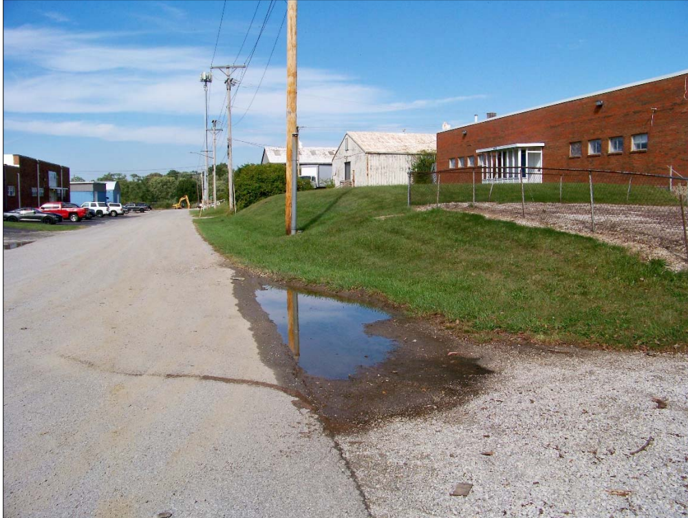
Poor drainage; no sidewalks in northwest corner of Area
