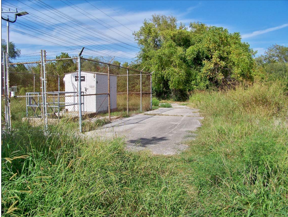
Deterioration of service drive at western edge of Area
