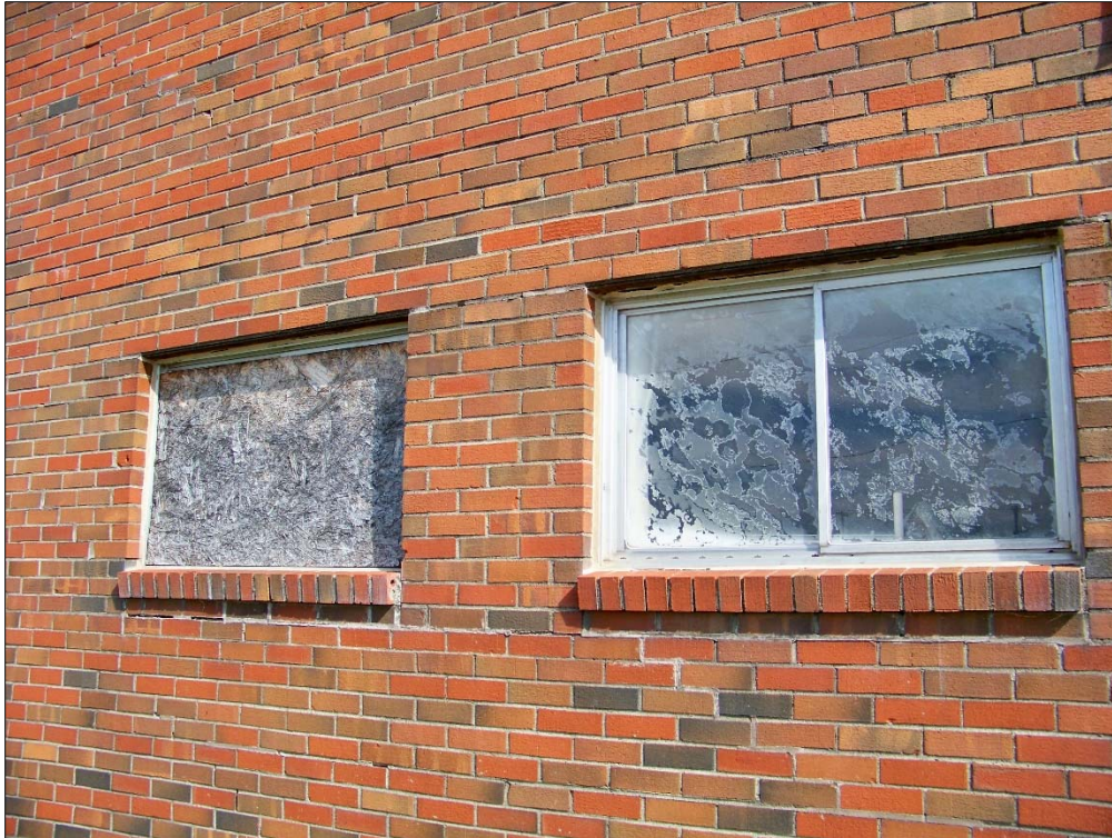
Deterioration of windows, lintels; need for pointing and repair of masonry at Weatherford Ave. building
