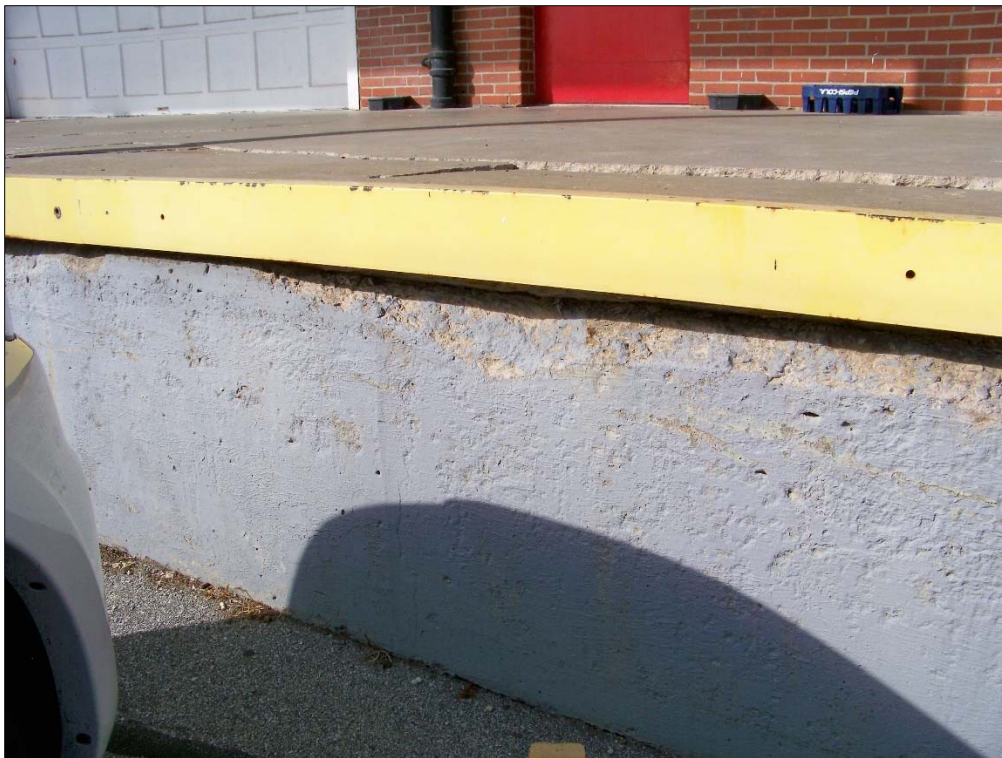
Deterioration of foundation of loading dock at Cargo Largo building
