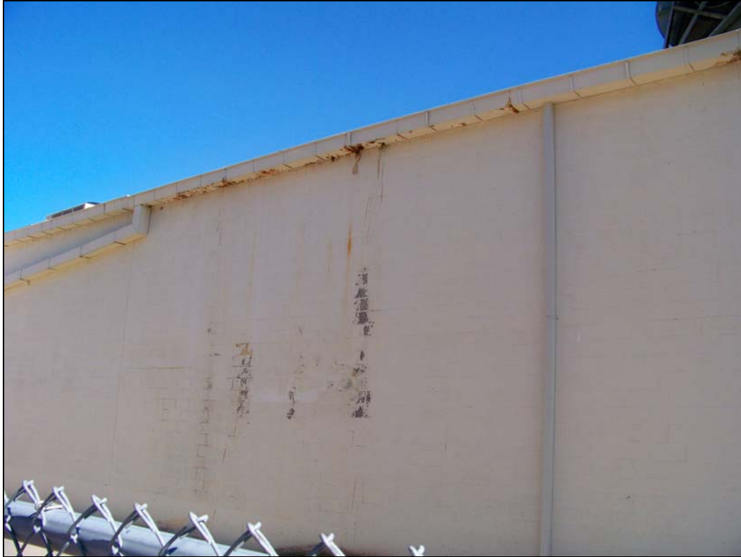
Building 1 – looking east – deterioration of gutter; failure of finishes
