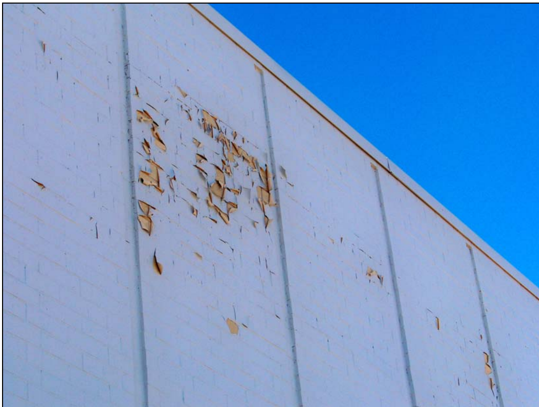
Building 1 – looking west – failure of finishes
