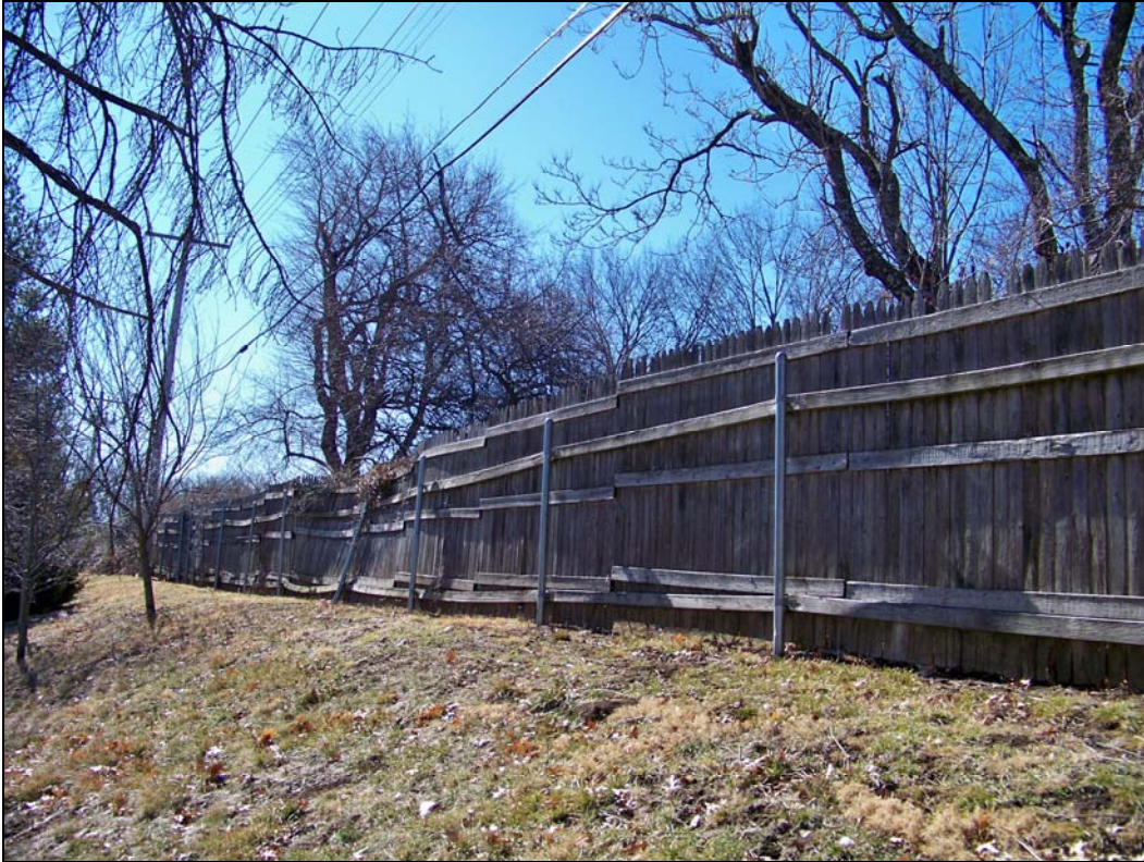
Near Building 1 – looking southwest – deterioration of fence
