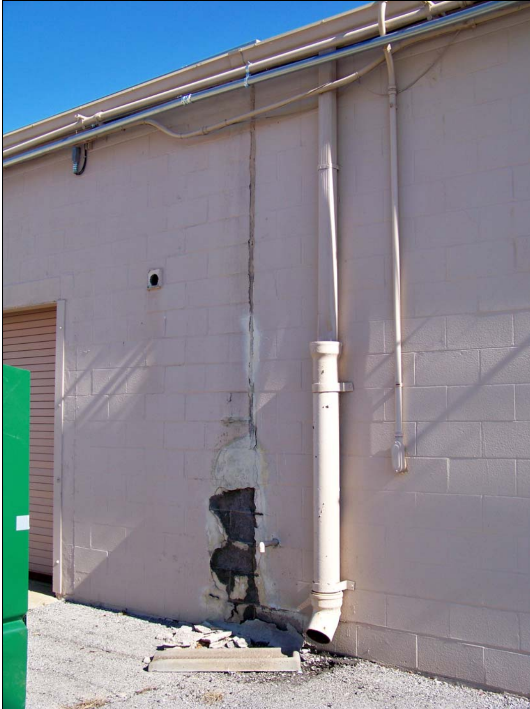
Building 1 – looking east – deterioration of downspout, wall; failure of finishes
