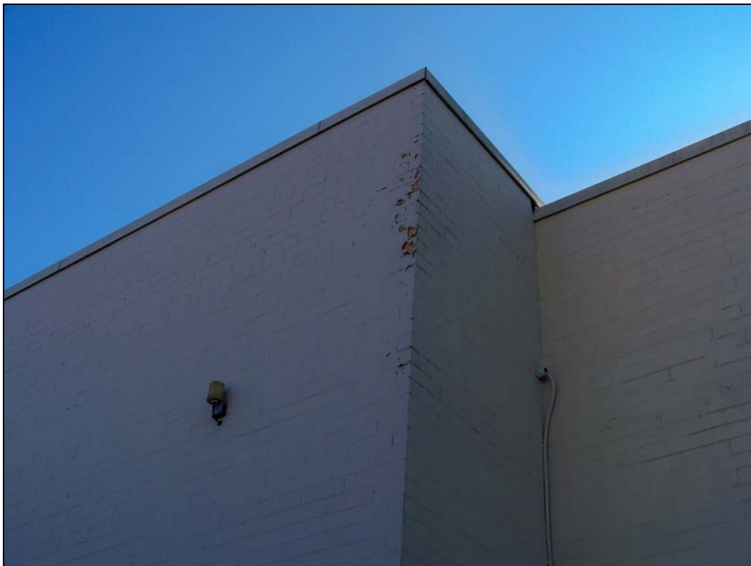
Building 1 – looking south – failure of finishes
