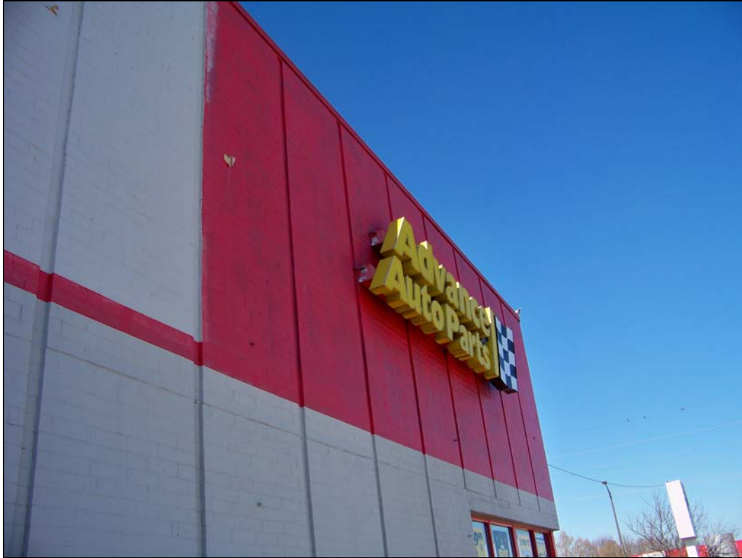
Building 1 – looking west – failure of finishes
