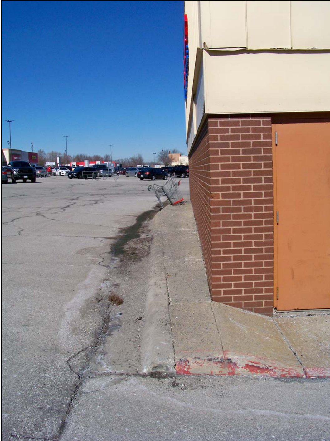
Building 2 – looking north – deterioration of pavement and sidewalk
