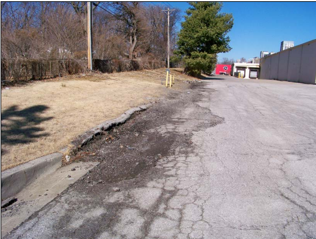
Near Building 1 – looking north – deterioration of pavement, curb
