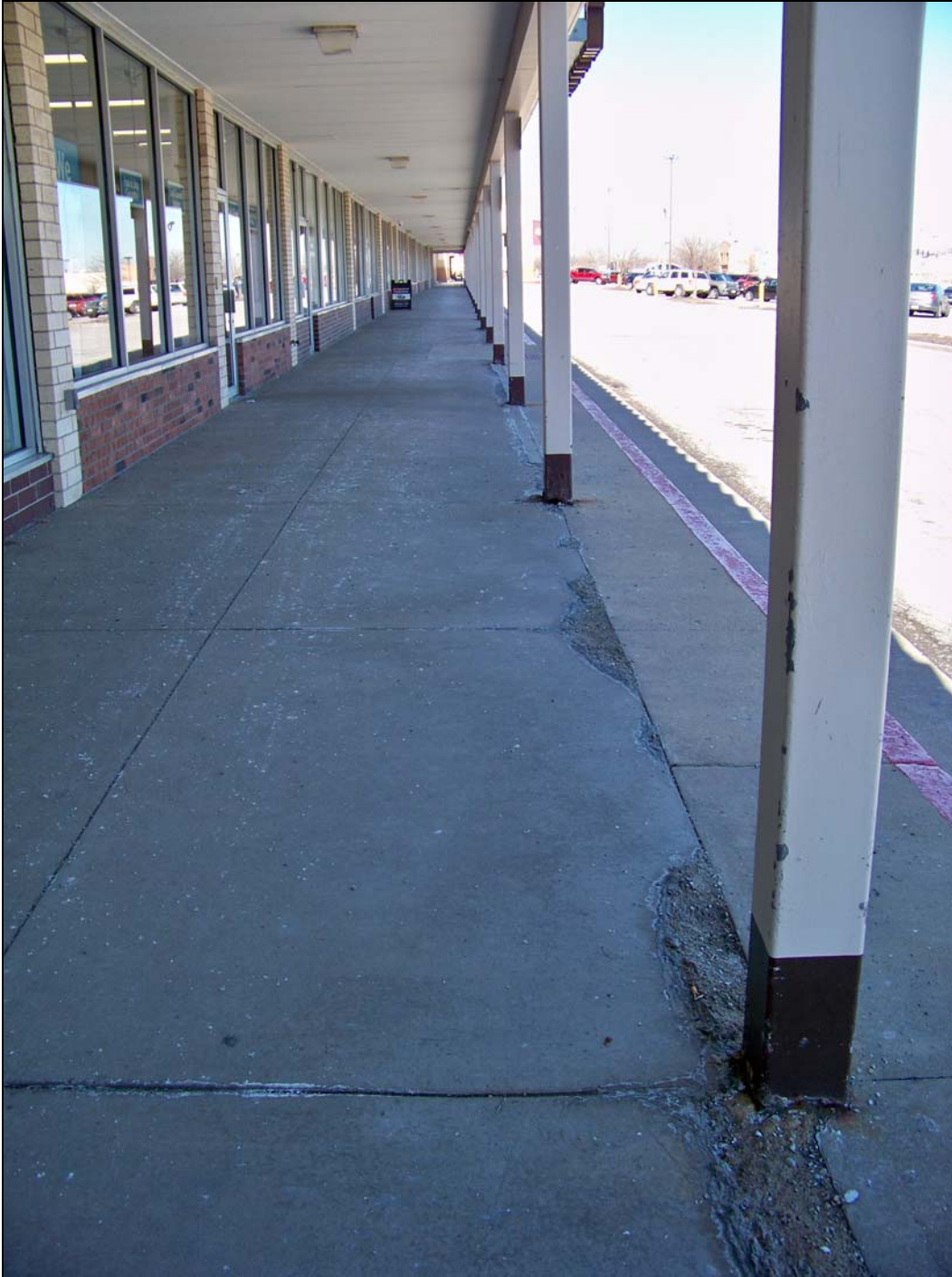
Building 1 – looking north – deterioration of sidewalk
