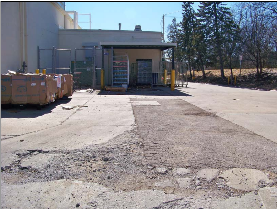
Building 1 – looking south – deterioration of pavement
