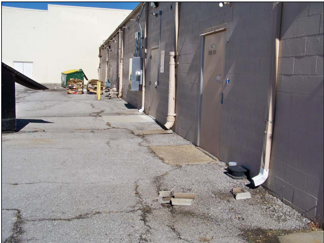
Building 1 – deterioration of downspouts, pavement; failure of finishes; unenclosed dumpsters
