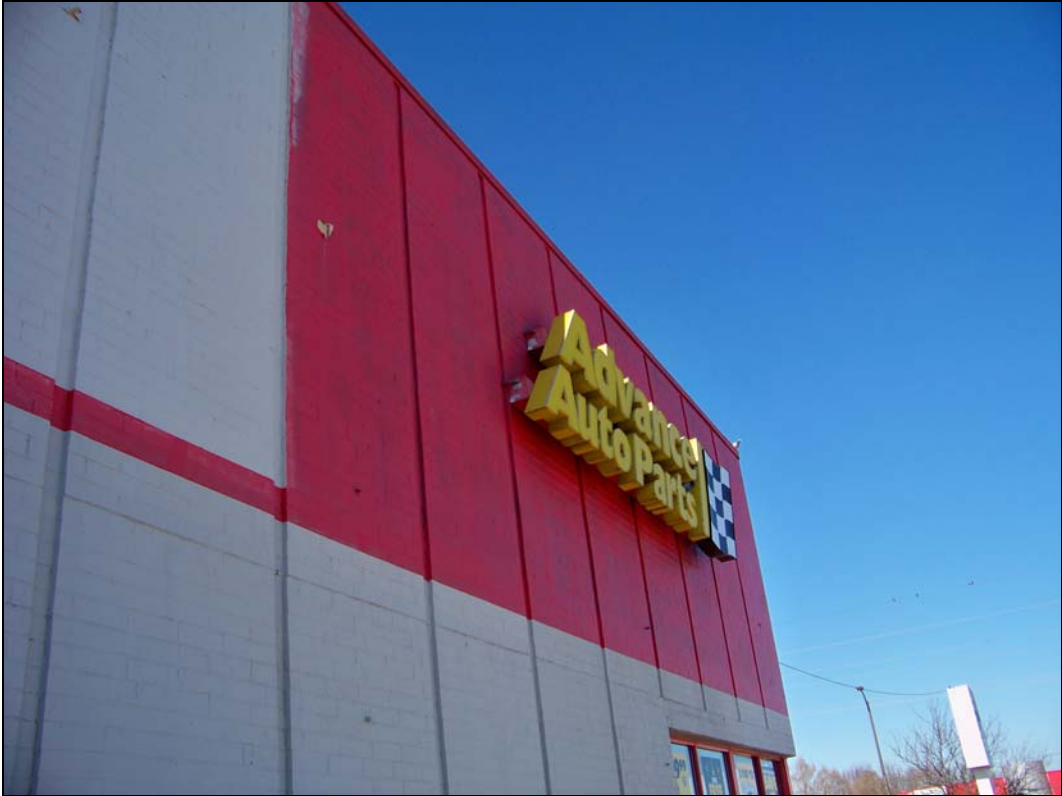
Building 1 – looking west – failure of finishes
