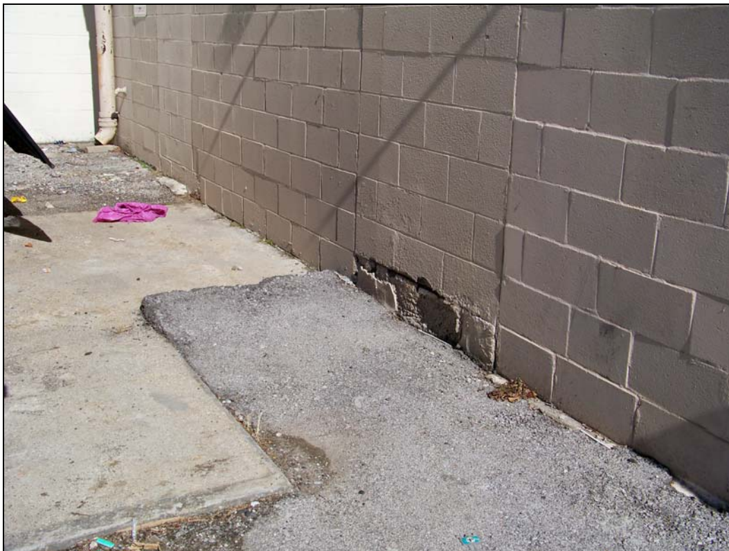
Building 1 – looking northeast – uneven pavement; deterioration of wall
