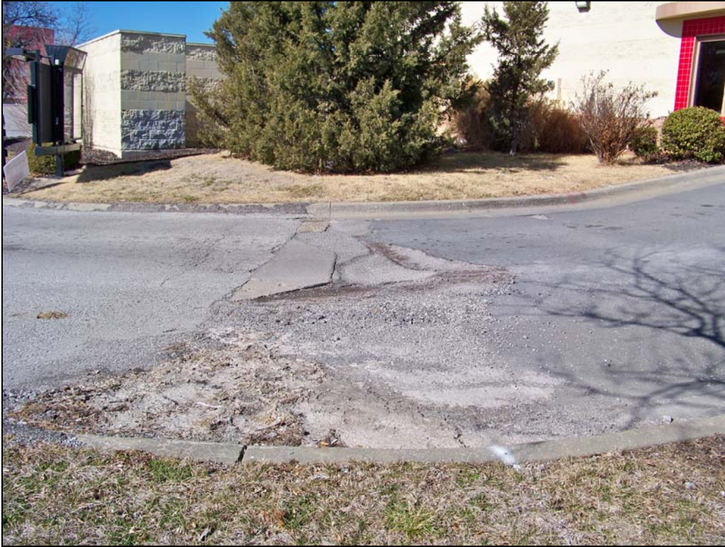
Building 3 – looking northwest – deterioration of drive aisle
