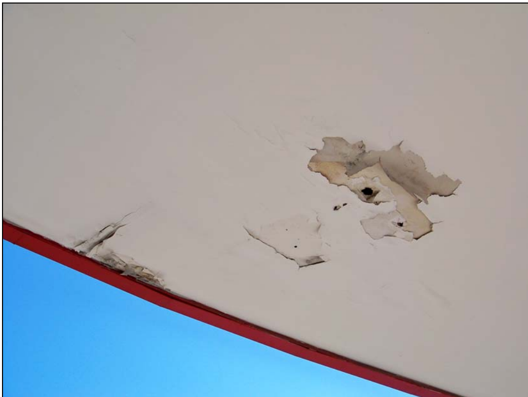
Building 1 – looking east – deterioration of soffit
