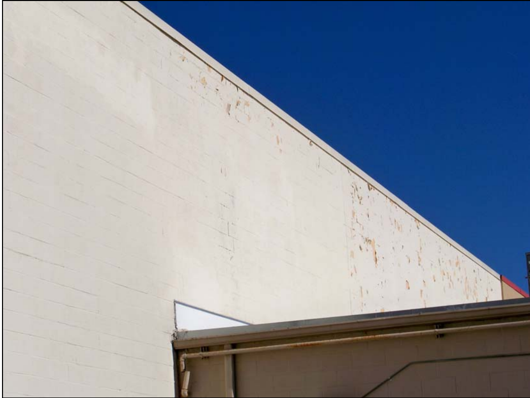
Building 1 – looking north – failure of finishes
