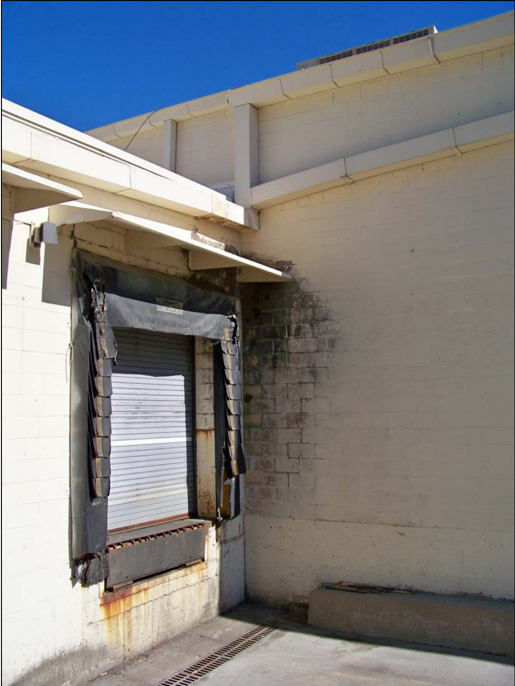
Building 1 – looking east – failure of finishes
