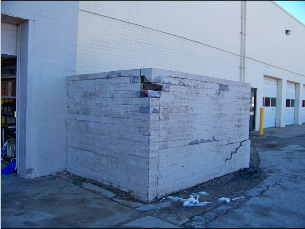
Building 1 – looking southwest – deterioration of trash enclosure, parking lot pavement
