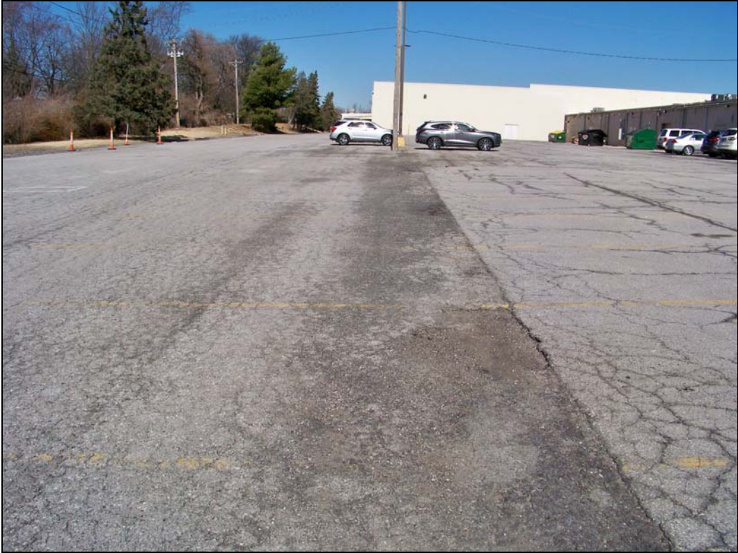
Near Building 1 – looking north – deterioration of pavement
