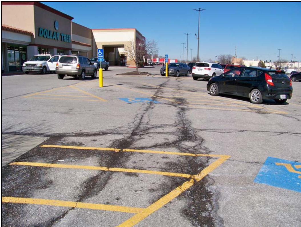
Building 1 – looking north – deterioration of parking lot
