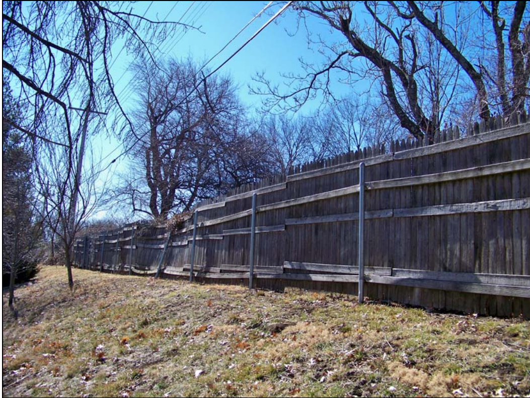
Near Building 1 – looking southwest – deterioration of fence
