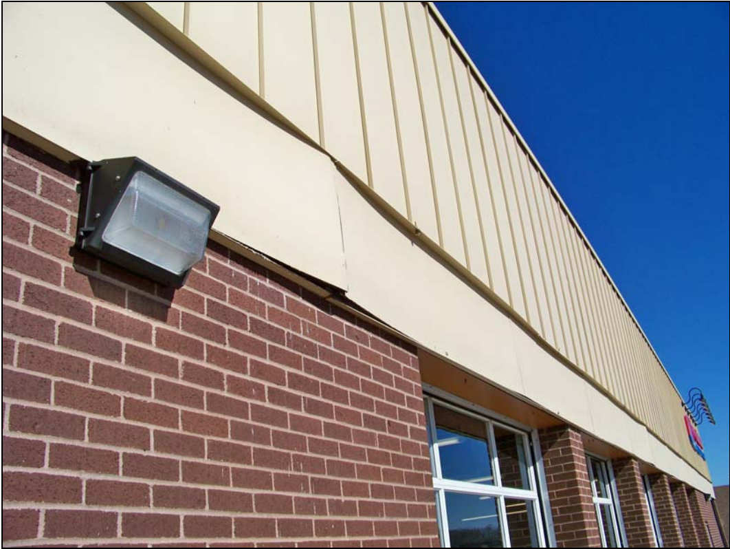
Building 3 – looking northeast – deterioration of fascia, siding
