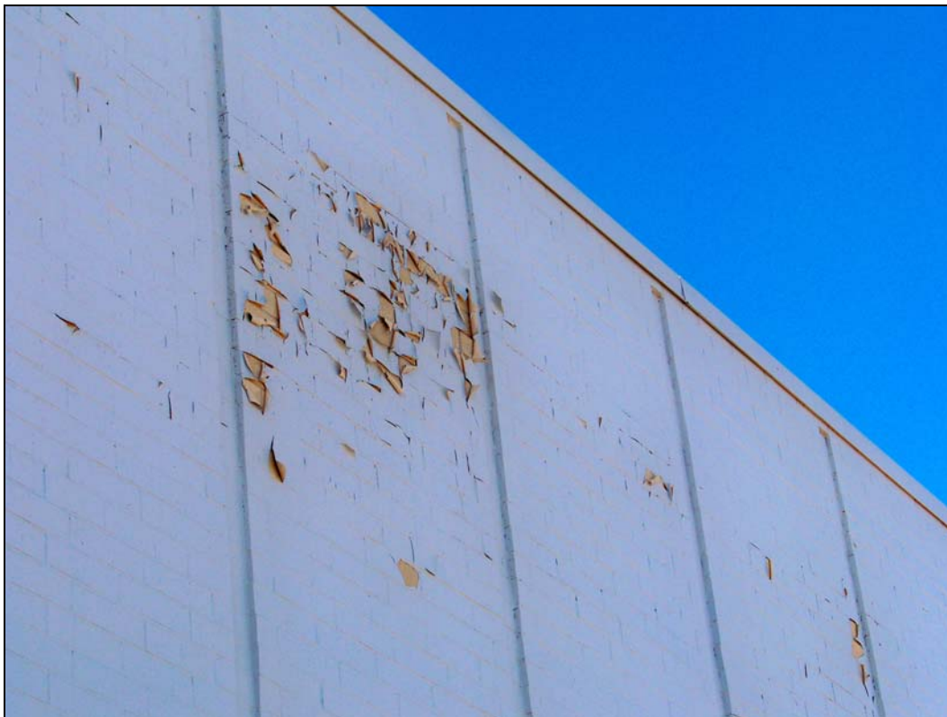
Building 1 – looking west – failure of finishes
