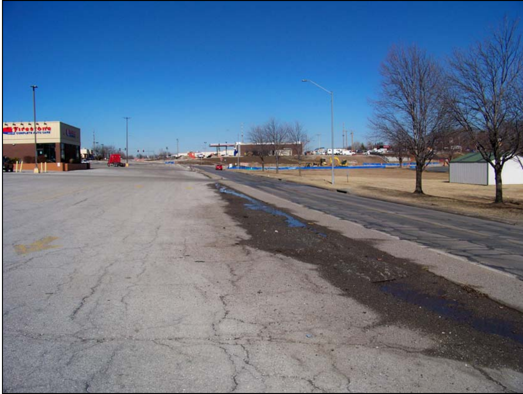
Near Building 3 – looking north – deterioration of parking lot; poor drainage
