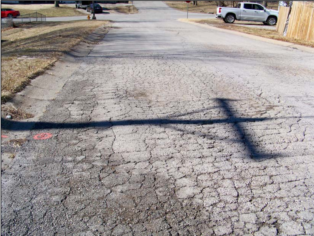
Near Building 1 – looking west – deterioration of driveway from Ellison Way
