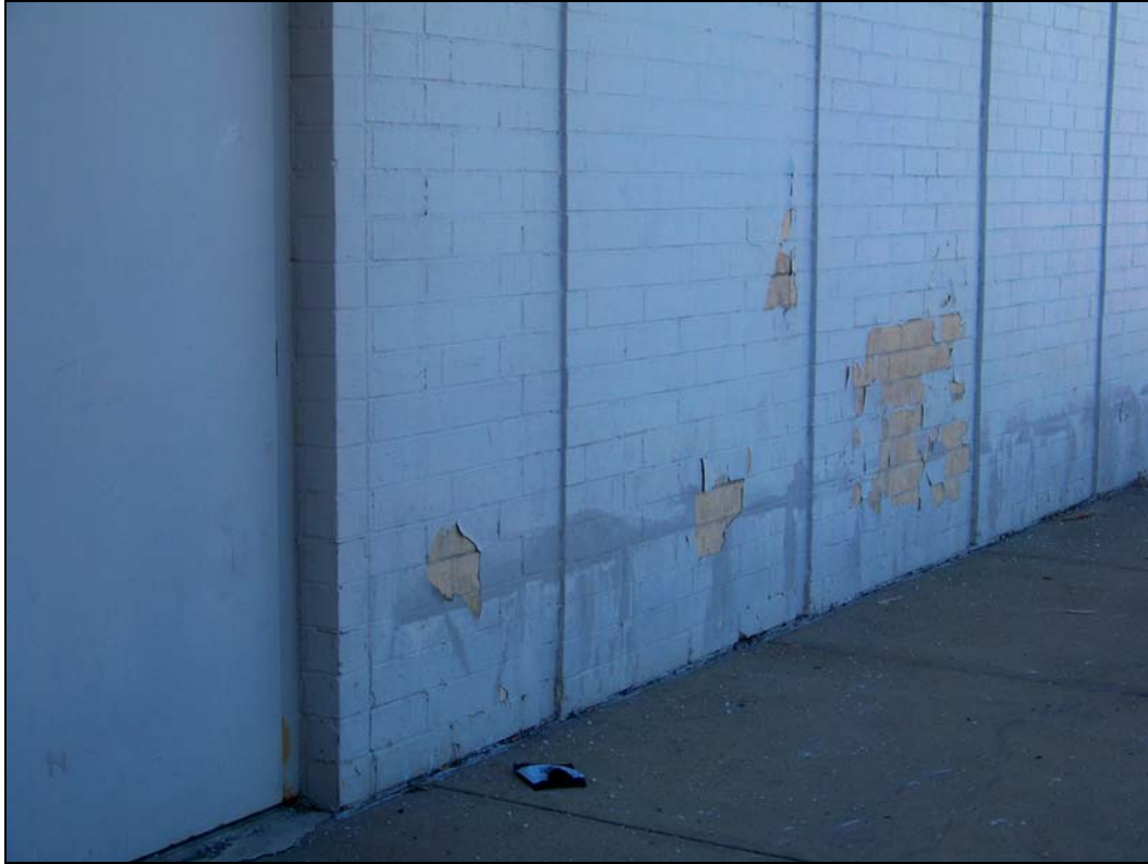
Building 1 – looking west – failure of finishes
